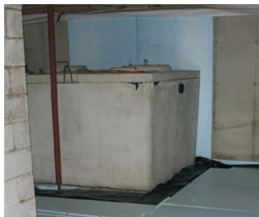
The concrete tank in the basement used for hot water storage. Right: Heat exchanger coils inside the tank. Below: The systems' mechanics wall, with the expansion tank, circulators, and boiler next to the PV system inverter and other electrical equipment.
