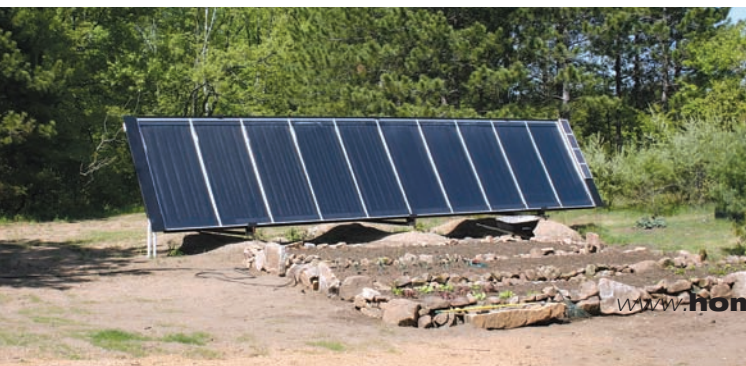
Solar collectors provide hot water for the house.
